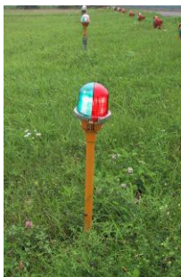
Fig. 8 Runway End/Threshold Lights
