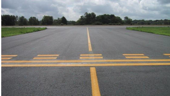
Fig. 5 Runway Holding Position Marking
